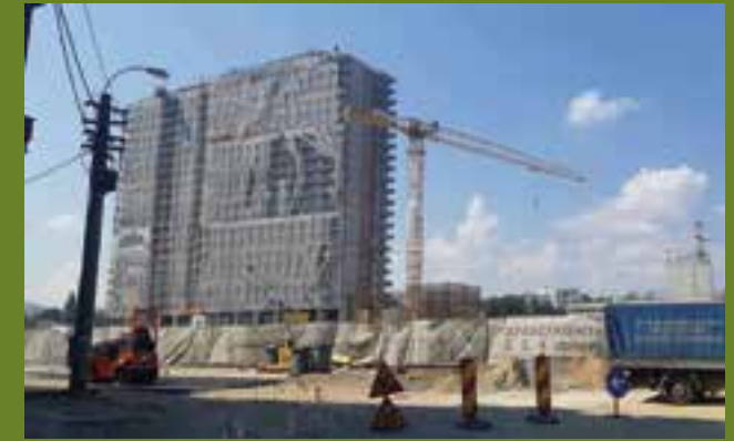
4. The new real estate developments on the spot of the former Abator slaughter house: the 23 story-building Maurer Panoramic (on the left: started in 2018, investor Maurer Immobiliare); Oxygen Assemble (on the right: Oxygen Mall and three 16 story-residential buildings, investor Mercurial SRL of a local businessman, with authorization from 2016).
